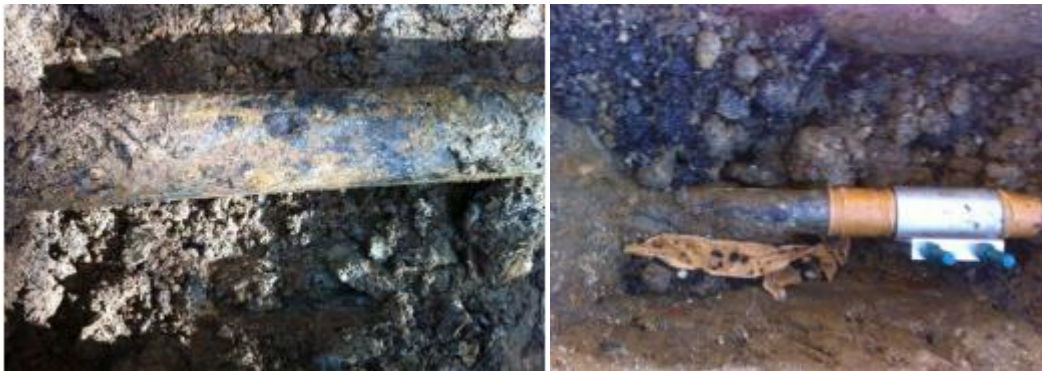
Figure 1-1&2: Examples of corroded cast iron mains and a repair clamp used throughout JGN
