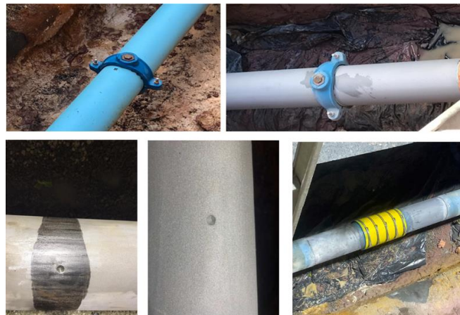
Figure 6–1: Chatswood Type A incident (Unauthorized Water Tapping Band)
