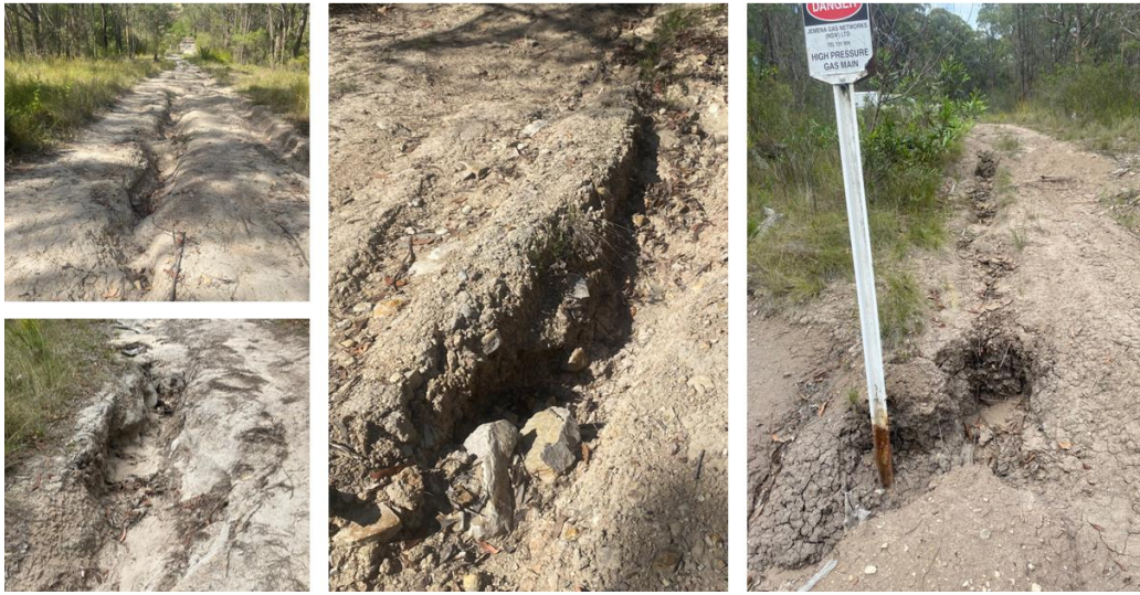
Figure 6–4: Gully erosion (Northern Trunk Wakefiled north of previous repairs) (prior to repairs)
