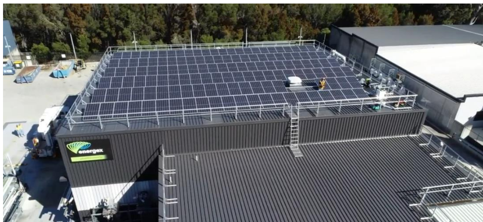
Image: Cleveland Depot Dynamic Solar PV Installation
