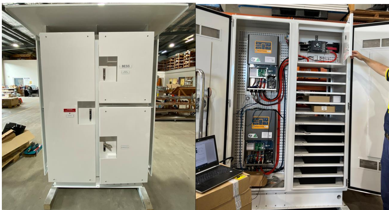
Images 5 and 6 - Inverters and rear of batteries during testing
