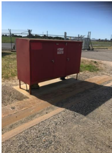
Figure 8: Typical Fire hydrant Booster
