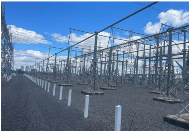
Figure 4: Typical switching yard image 1
