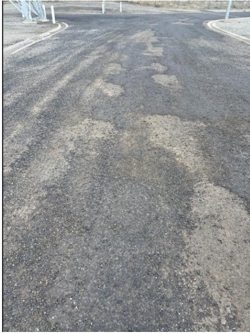
Figure 26: Poor condition of Roads at SMTS
