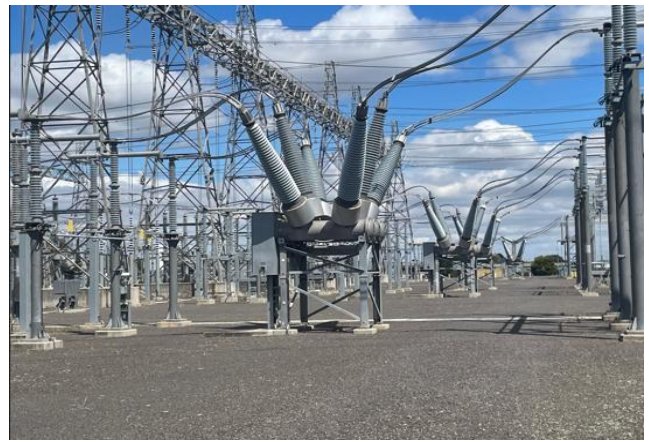
Figure 5: Typical switching yard image 2
