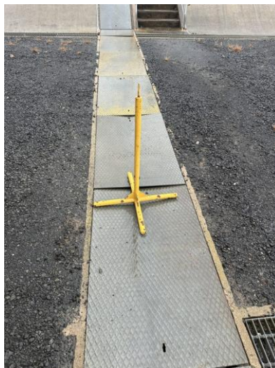
Figure 25: Poor condition of cable trench covers at BETS
