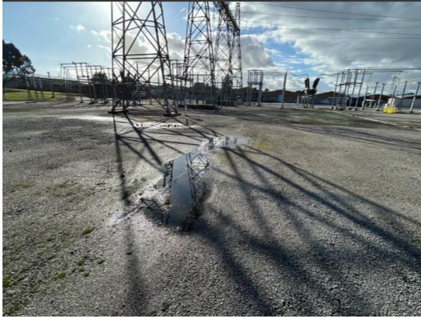
Figure 24: Poor condition of Switchyard at HTS
