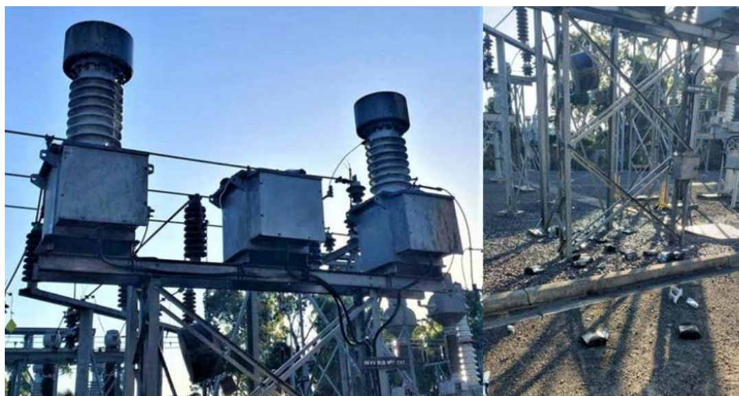
Figure 19: [ C.I.C ] CVT failure in 2022
