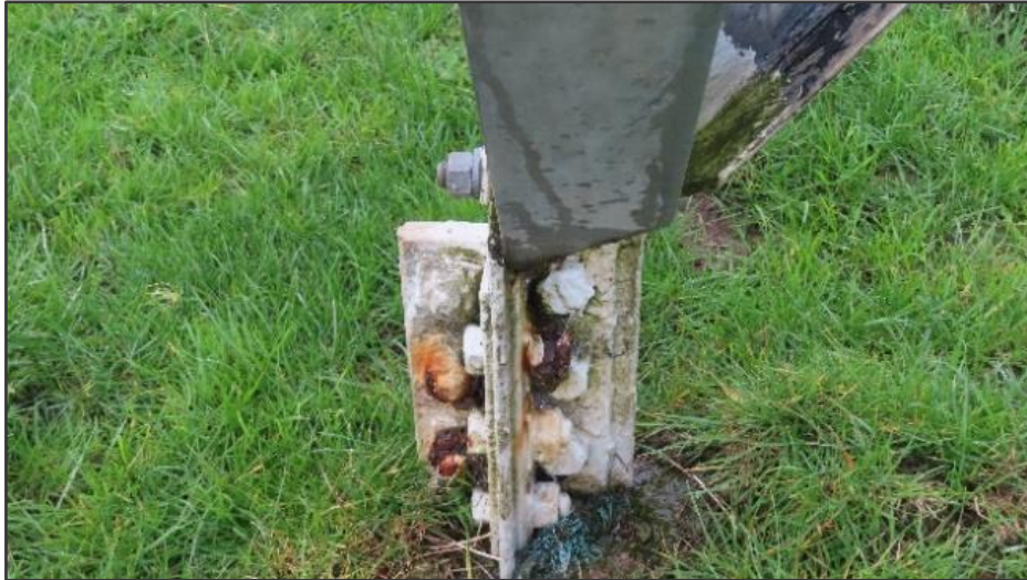
Fig 18: Damaged SOXS, T197 MLTS-TGTS 220kV
