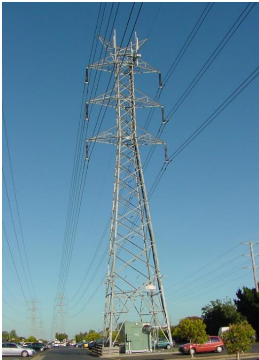
Figure 65: ROTs-SVTS 220 kV suspension tower
