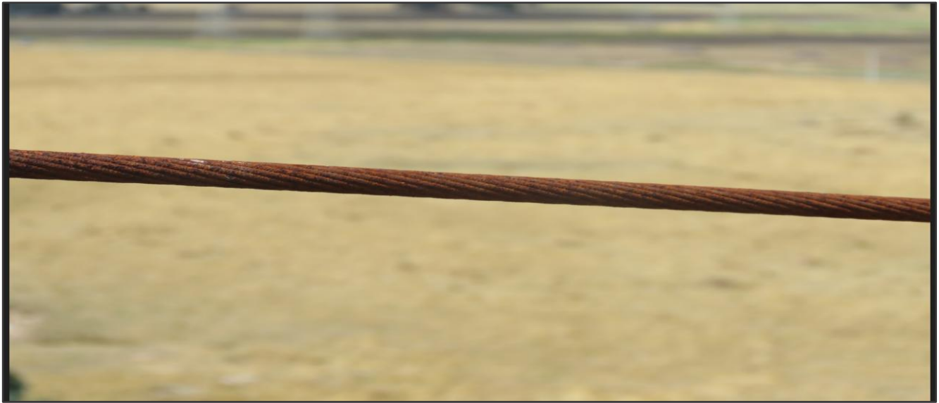
Figure 8: Corroded Steel Ground Wire rated as condition C4
