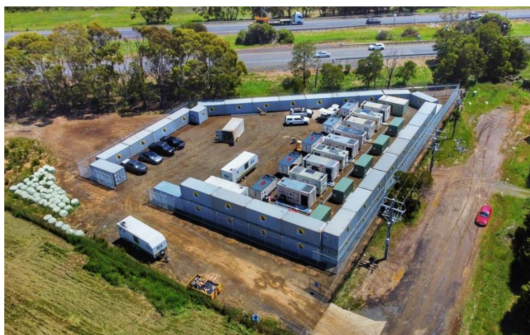
Figure 5-13: Temporary Generator Site at Wallan (for KLO14 and KLO24)
