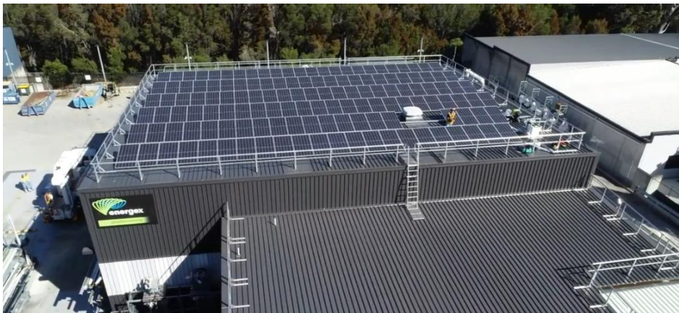
Figure 1 - Cleveland Depot Dynamic Solar PV Installation
