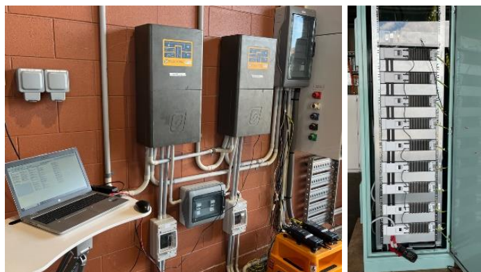
Figure 8 – SAPS and Polarium Battery Testing
