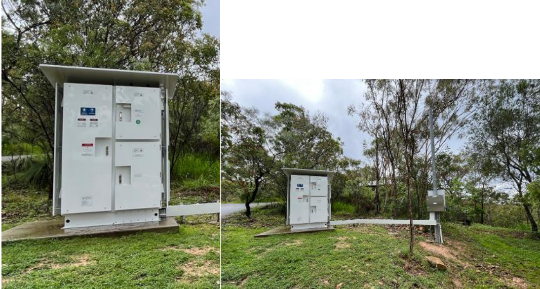
Figure 12 - The BESS cubicle onsite at the Allawah retreat
