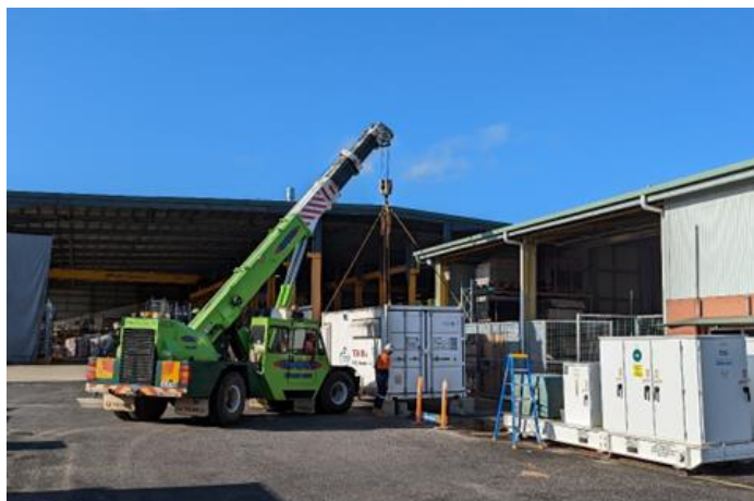
Figure 10 - Centralised Energy Storage System
