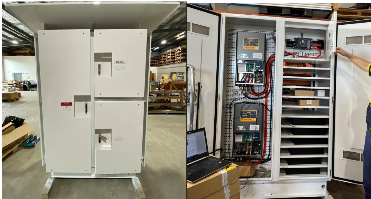
Figure 11 - The Project Cubicle, Inverters and Batteries during factory testing
