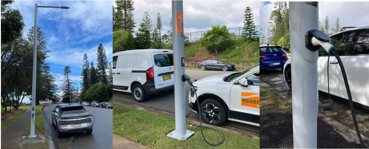
Figure 3: Composite streetlight in-asset charger – First of its kind 7kW AC charger
