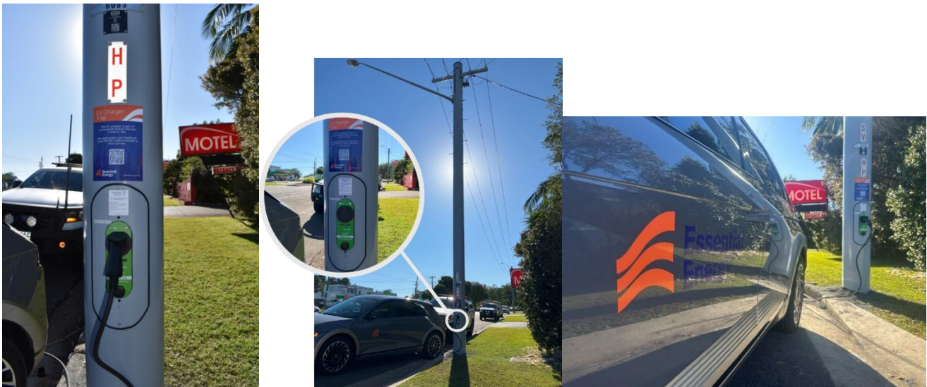
Figure 4: Composite distribution pole in-asset charger – First of its kind 22kW AC charger
