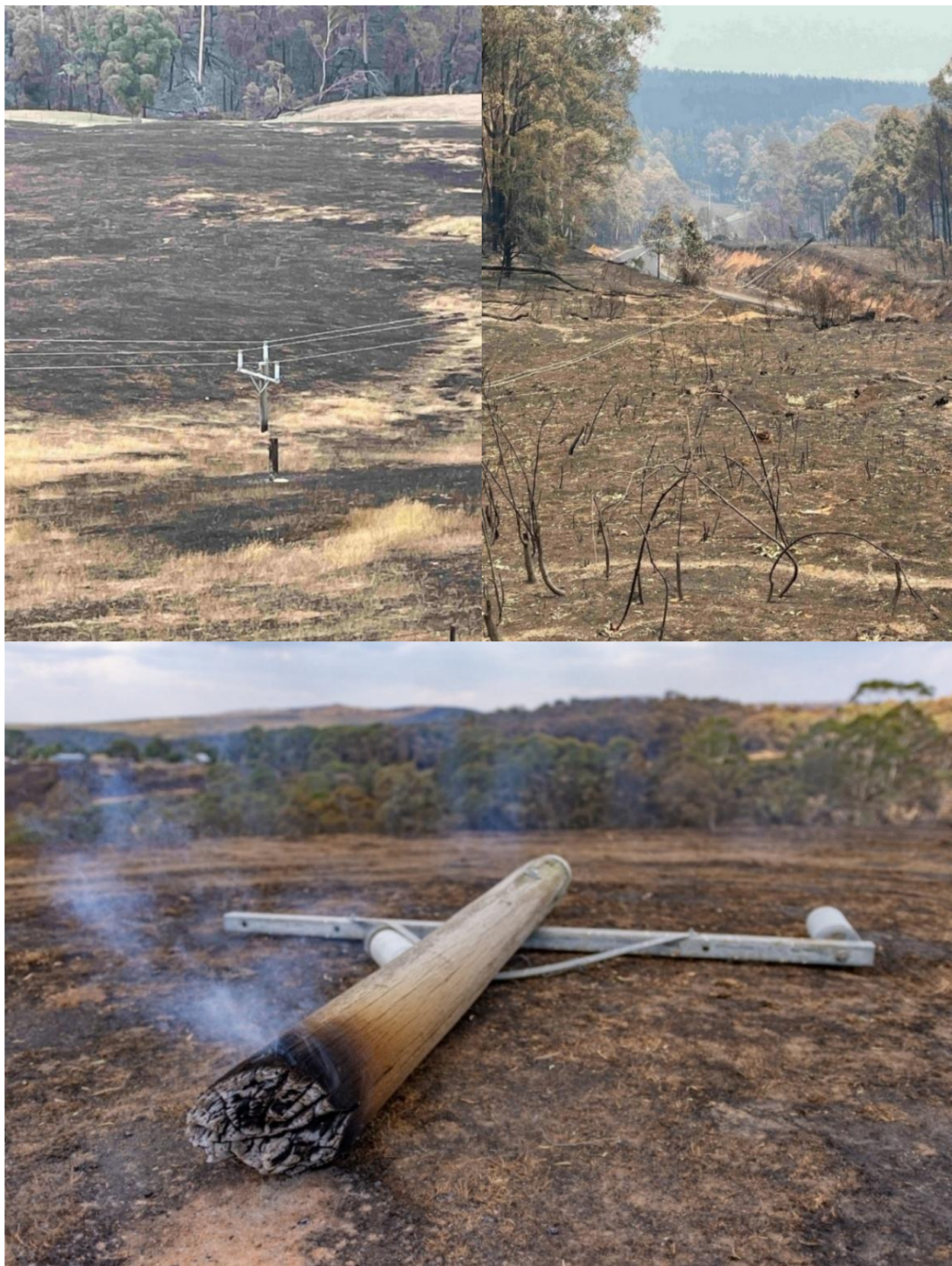
Figure 5: Examples of severe damage to our network as a result of the January Walwa bushfire along Murray Valley Hwy, Koetong. 15
