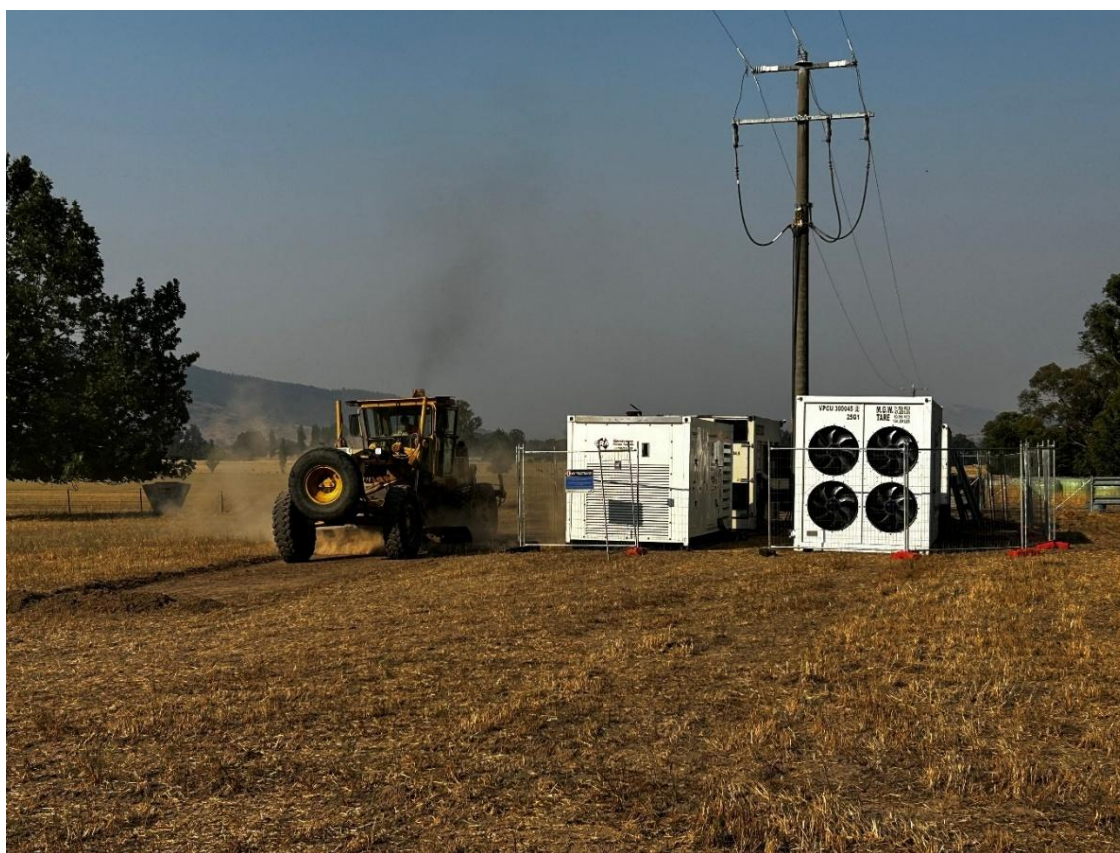
Figure 10: Temporary generators installed to restore customer supply for Corryong township.
