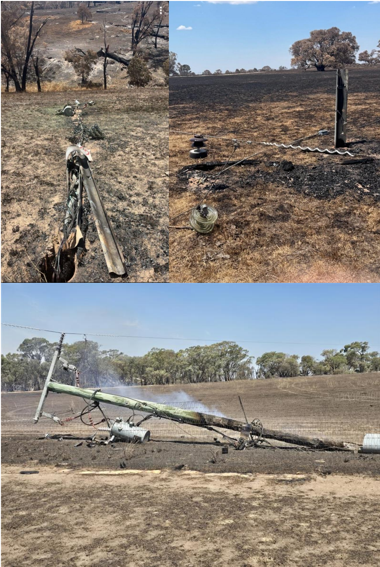
Figure 6: Examples of severe damage to our network as a result of the January Longwood bushfire in the Highlands. 16
