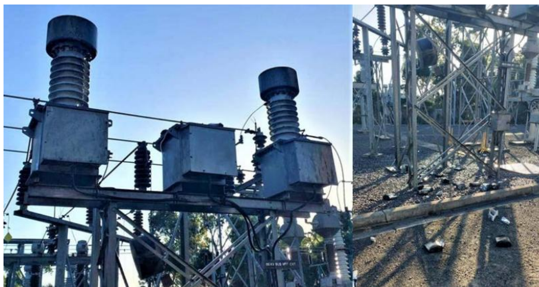
Figure 19: [ C.I.C ] CVT failure in 2022
