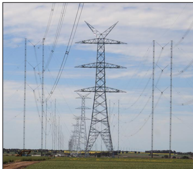
Figure 33: A 500kV tower with ERS bypasses on either side of the tower
