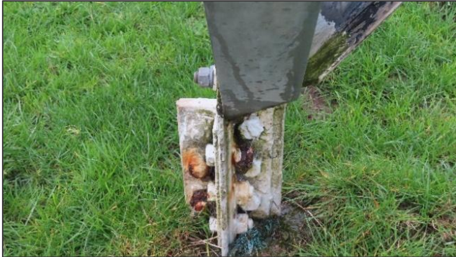
Fig 18: Damaged SOXS, T197 MLTS-TGTS 220kV
