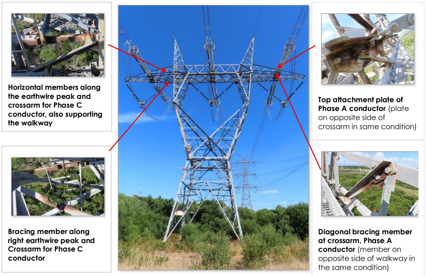
Figure 26: T628B, corrosion of plates and interconnected members
