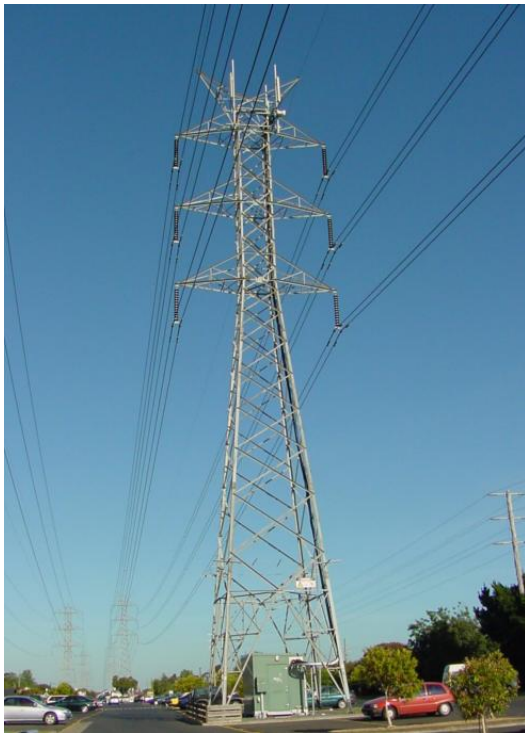
Figure 65: ROTS-SVTS 220 kV suspension tower
