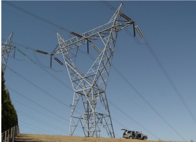
Figure 54: DDTS-SMTS No. 1 330 kV strain tower
