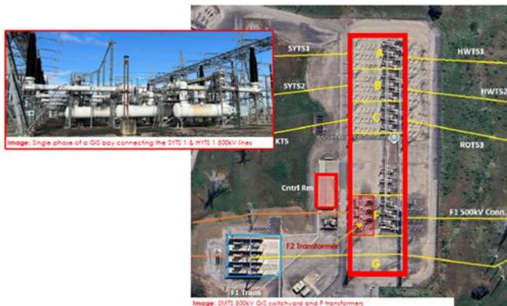
Figure 4.6: Location and condition of SMTS 500kV GIS
