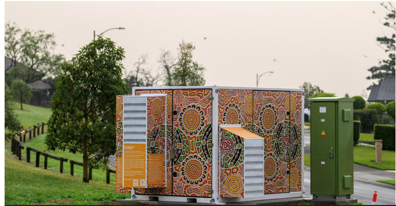
Image: Blair Athol Battery Energy Storage System Artwork by Indigenous Artist, Jenny Shillingsworth
