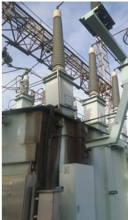
Figure 1: 1992 [C-I-C] bushings with oil leak
