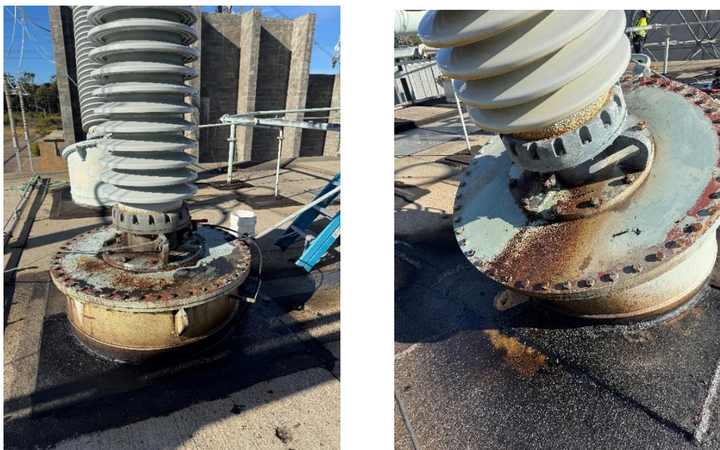
Figure 2: 1989 [C-I-C] bushings with oil leak and corrosion
