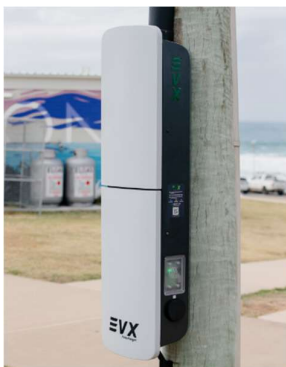
Figure 1: Example of EVCI installed on a distribution pole
