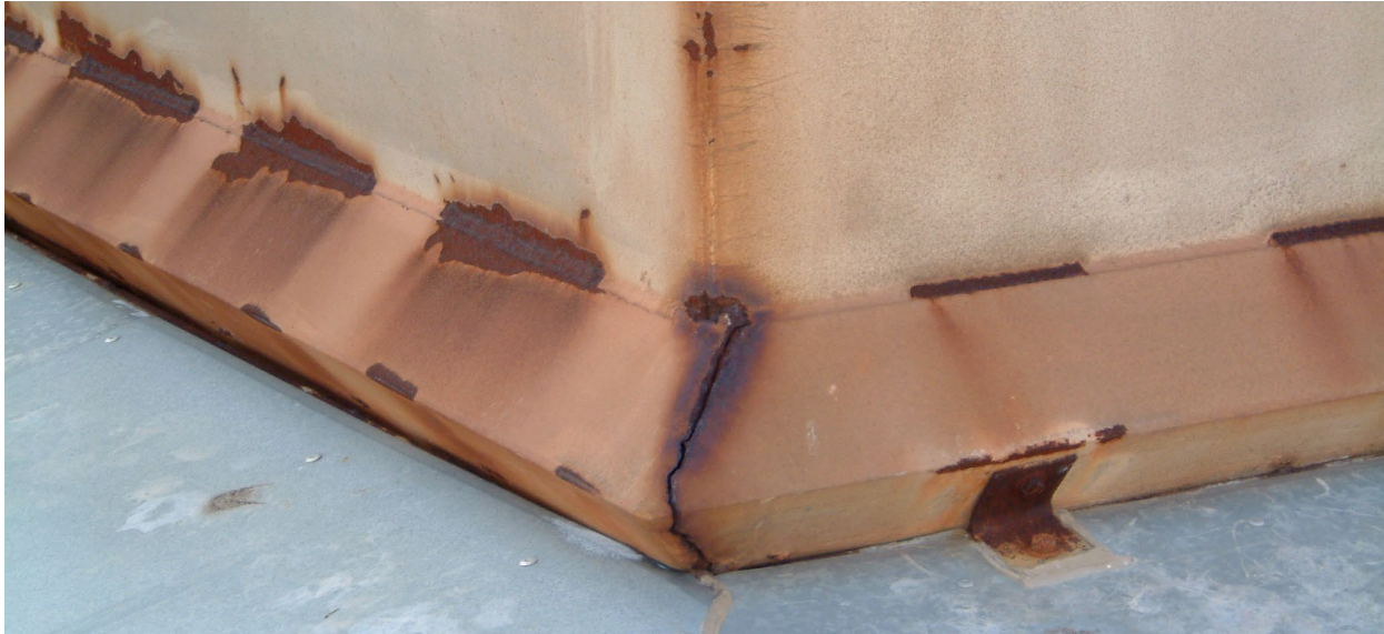
Figure 1 - Exhaust stack cracking
