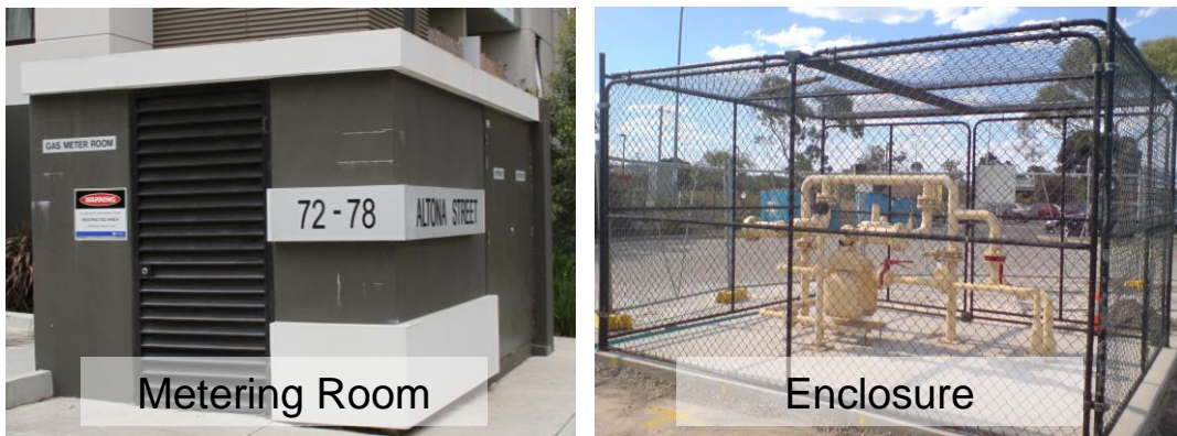
Figure 7: Metering Room and Enclosure
