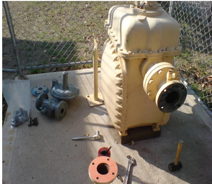
Figure 13: I&C regulator undergoing Full Overhaul
