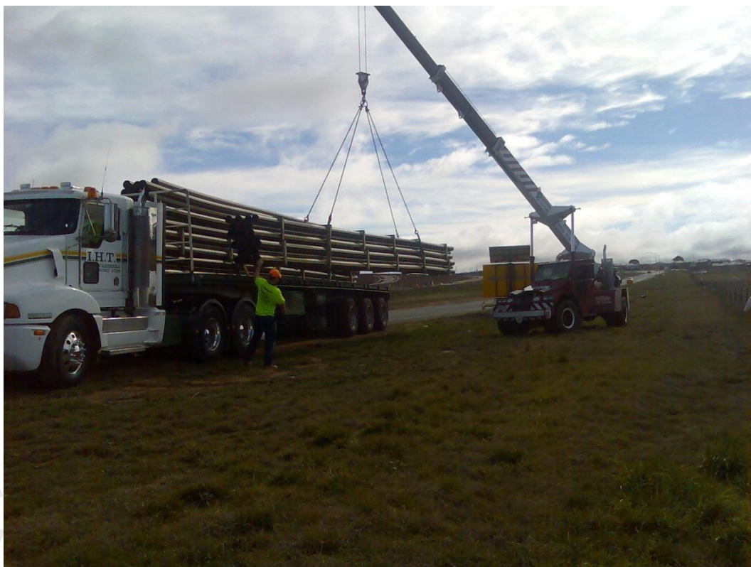
Figure 9–4: PE pipe for feeder main to supply gas to the new suburbs of Jacka and Moncrieff.
