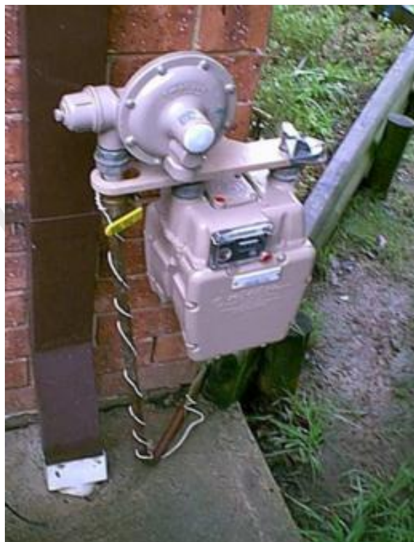
Figure 12–7: Typical residential gas meter
