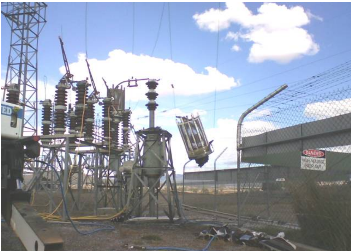
Figure 3 - Explosive failure of a Ducon 110 kV voltage transformer at Avoca Substation
