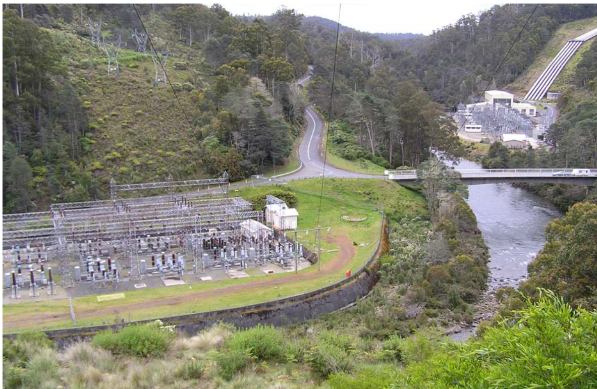
Figure 2 – Image of existing Tarraleah Switching Station (left) and Tungatinah Substation (right)
