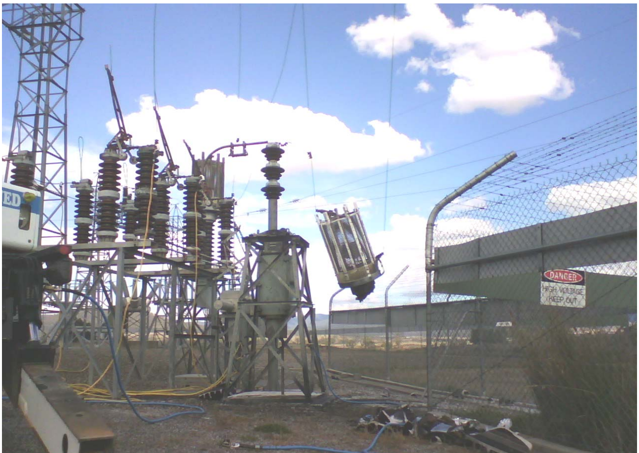
Figure 3 – Explosive failure of a Ducon 110 kV voltage transformer at Avoca Substation (March 2008)
