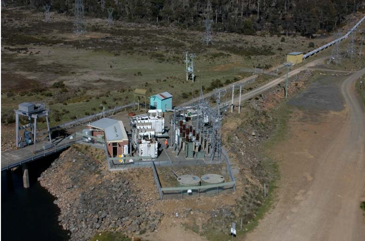
Figure 2 – Aerial view of Arthurs Lake Substation
