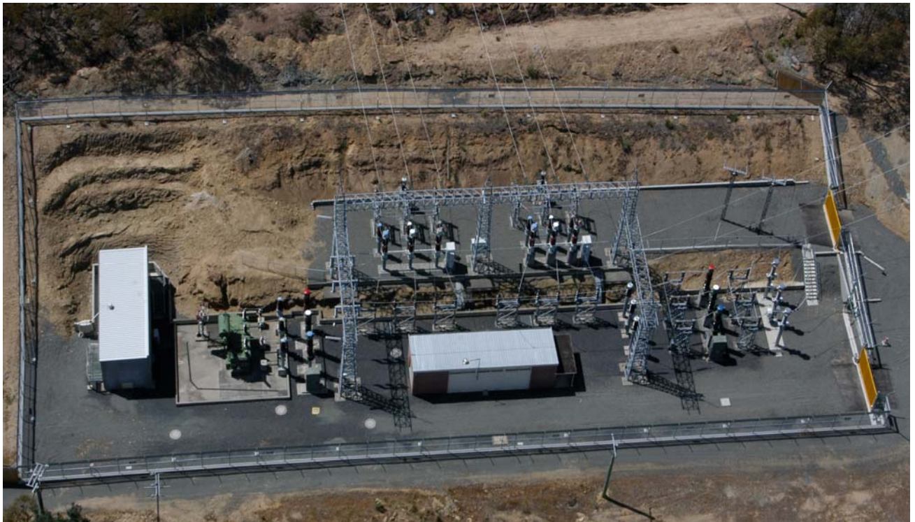
Figure 1 - Aerial view of Meadowbank Substation
