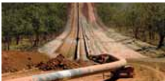
Bonaparte Gas Pipeline
