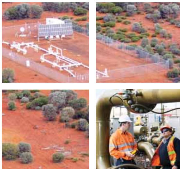
IMAGES: (from top) Goldfields Gas Pipeline scraper station, Western Australia; Michael Mann and Attila Csizmadia at Brooklyn city gate, Victoria
