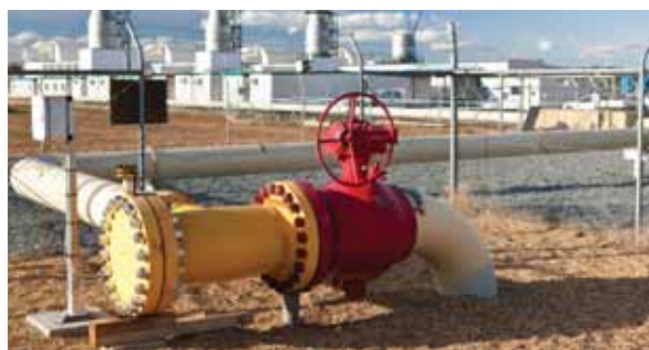
IMAGE: Gas delivery to Uranquinty Power Station, New South Wales.
