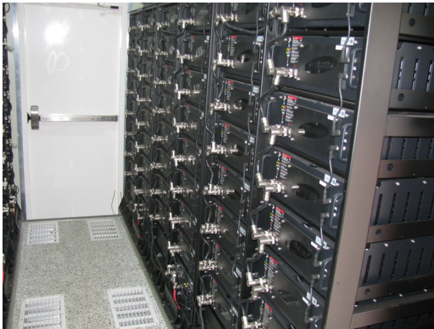
Figure 5.2 Battery container view from inside.
