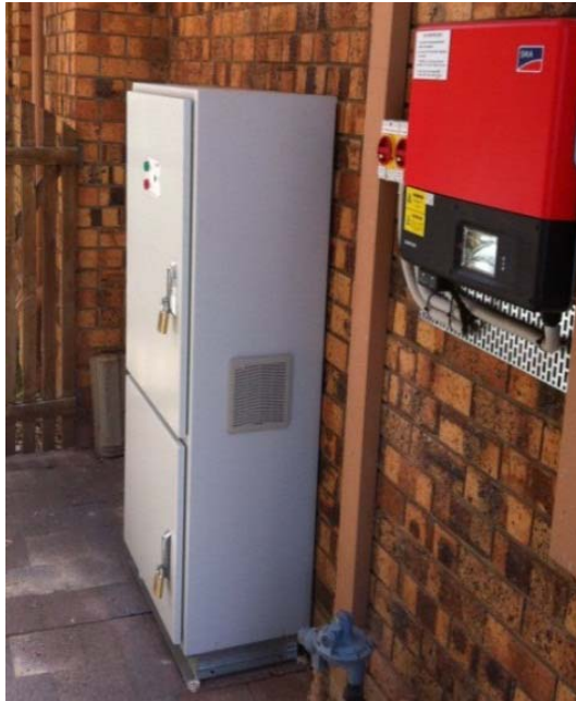
Figure 4.1 An installed Residential Battery Storage System (batteries in lower compartment of cabinet, inverter/charger and control system in upper compartment), and wall-mounted solar inverter.
