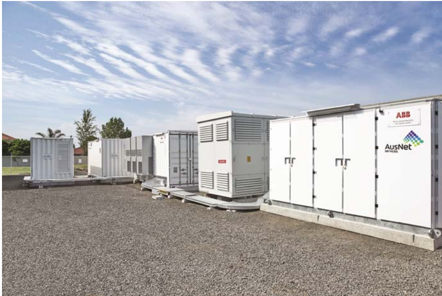
Figure 5.1 The GESS, installed and operational. Battery containers are in the background, with the inverter, transformer and switchgear containers in the foreground.
