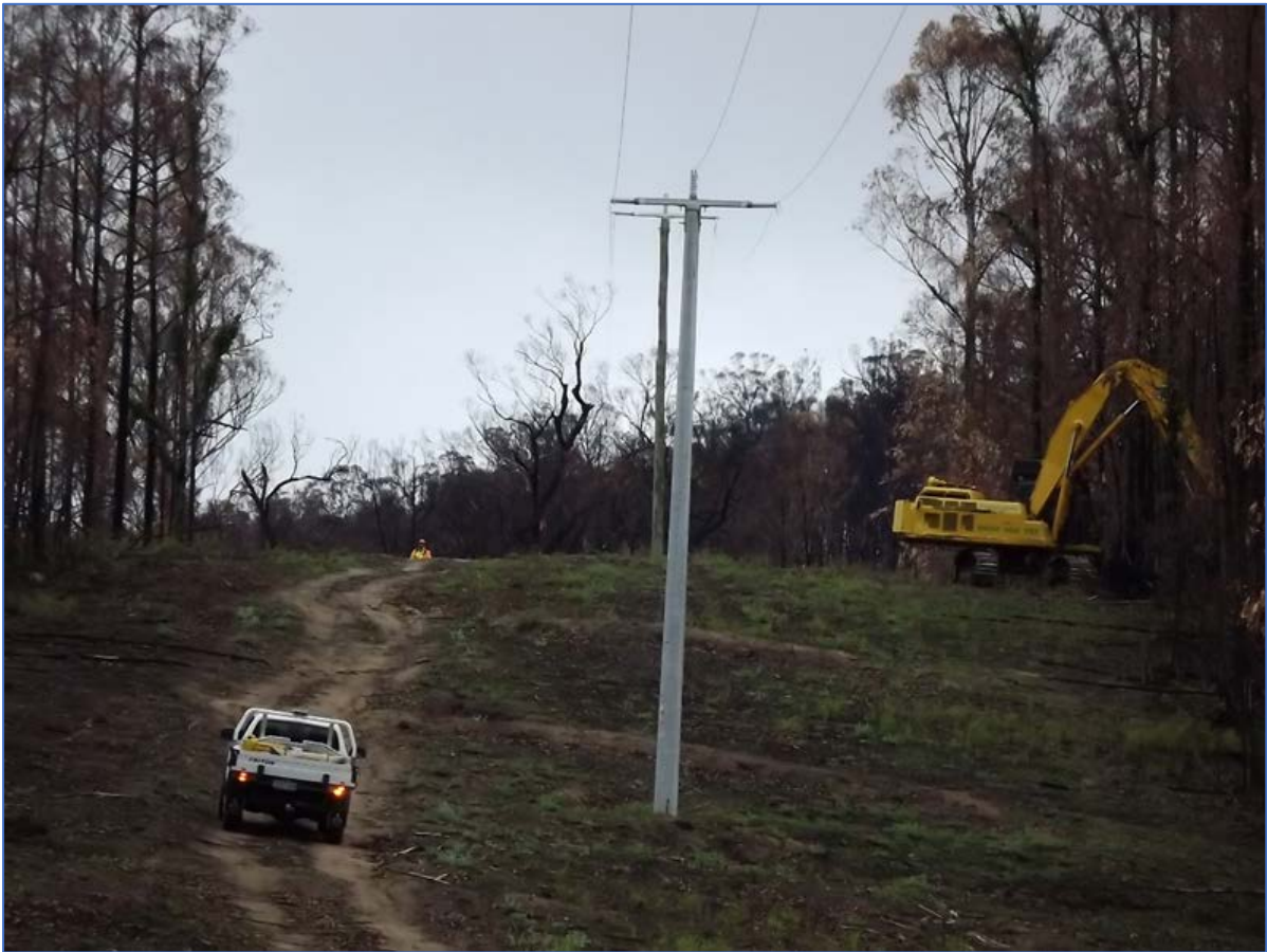
Figure 9: Hazardous trees adjacent to the powerline being removed
