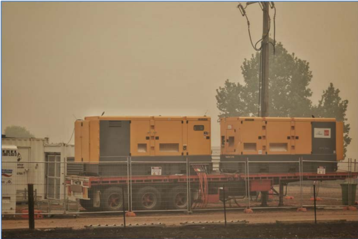
Figure 6: Temporary generators installed to restore customer supply at Corryong
