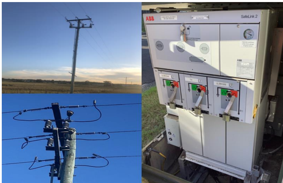
Figure 11: 11kV air break switch (left) vs 11kV ring main isolator switch (right)
