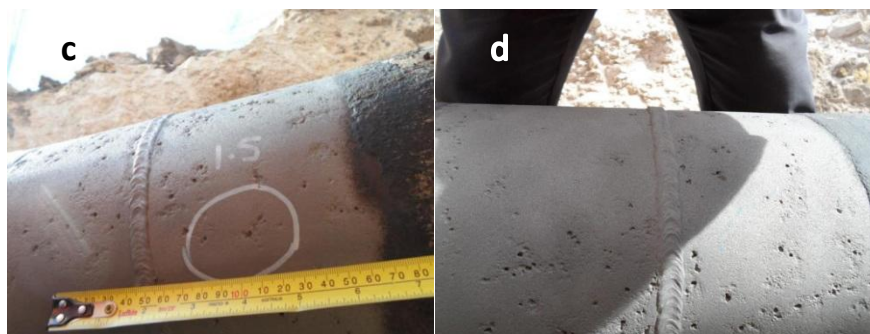
Figure: Photos taken from HSS excavation sites of M21 and M53 pipelines, showing deep tunnelling pits (a and b) scattered (c and d) over pipe surface.
