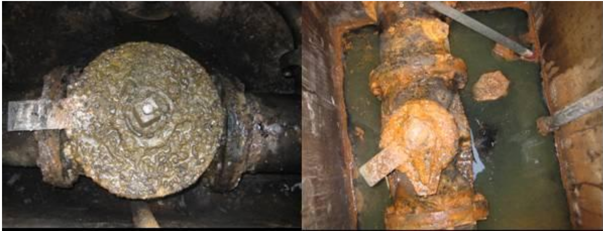
Figure 1: Isolation Valves located in Vaults - Examples
