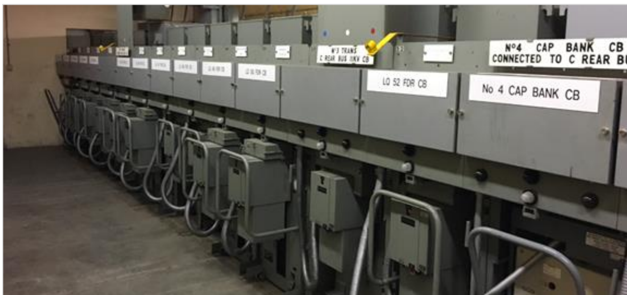
Figure 4.7 Little Queen zone substation: 11kV switchgear
