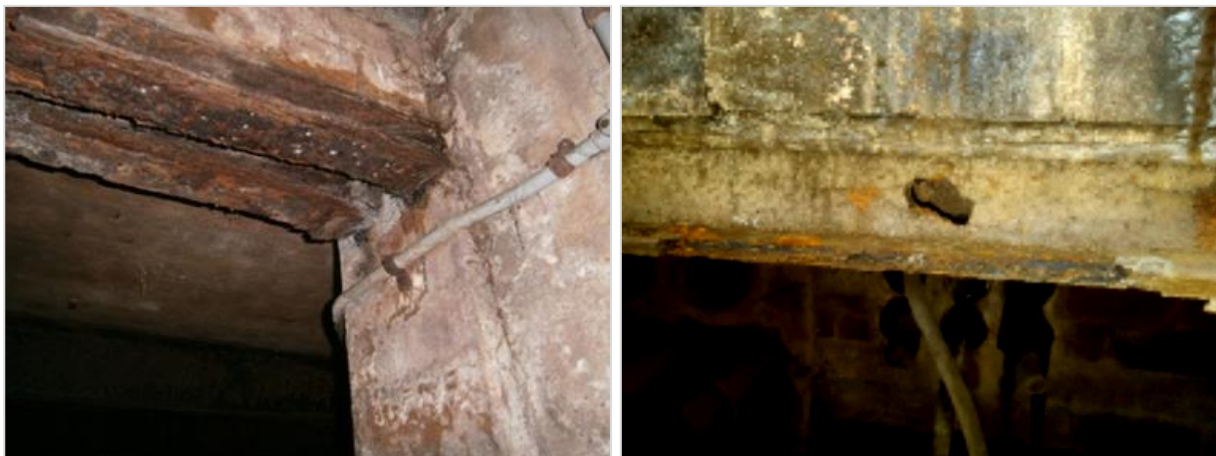
Figure 4.9 Corrosive damage to supporting steel work inside CBD cable pits
