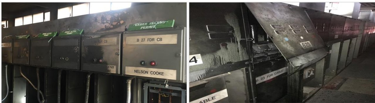
Figure 4.8 Damage to busbar chamber and switch room due to explosive failure at Collingwood zone substation (2016)
