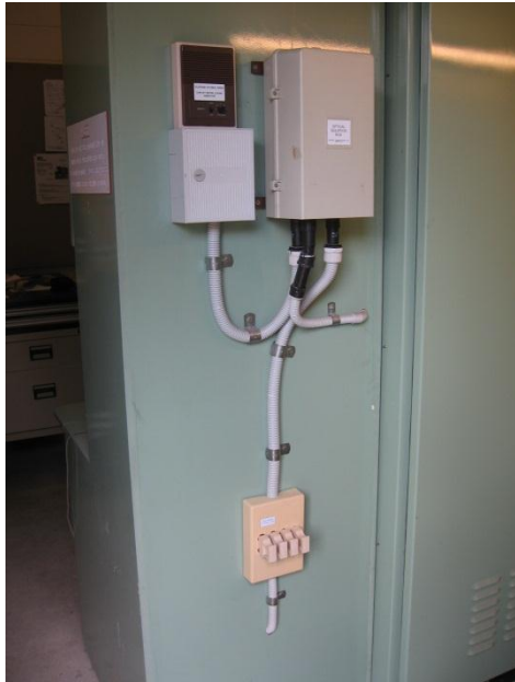
Figure 5: Non- Compliant isolation – Close Proximity to earthed metalwork (adjacent cabinet)
