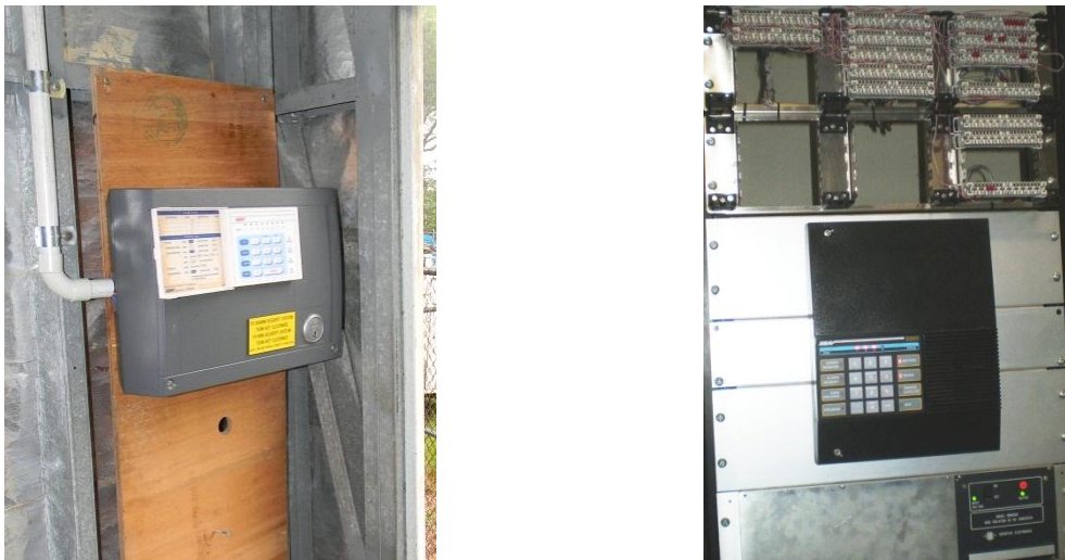
Figure 7: Typical remote site security panels
