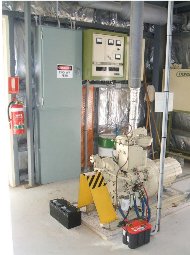
Figure 1: Typical remote site diesel generator
