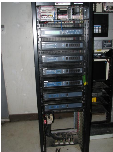
Figure 3: Solar Regulators – D'Aguilar Range Repeater
