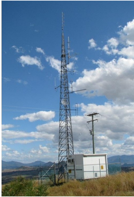
Figure 4: Typical Telecommunications Radio Tower
