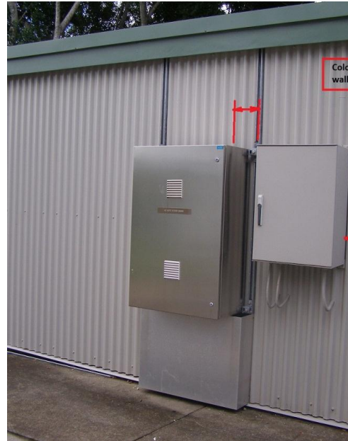
Figure 6: Isolation cabinet mounted on metal sheeting, and close to GPO and other equipment
