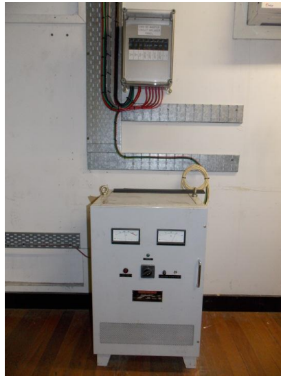
Figure 2: Raceview Depot battery charger – estimated manufacture date 1989
