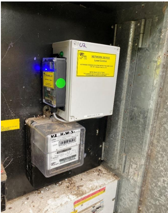
Image 1: Load control relay and comms device in-situ
