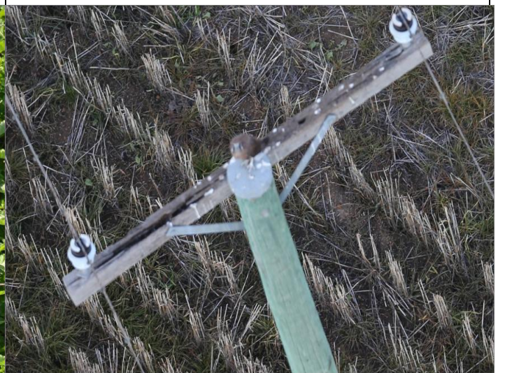
Large crack and hole in end of crossarm – A3 task
