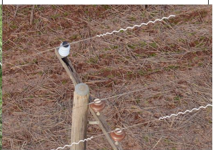
Crossarm deteriorated, hole in end of arm – A3 Task
