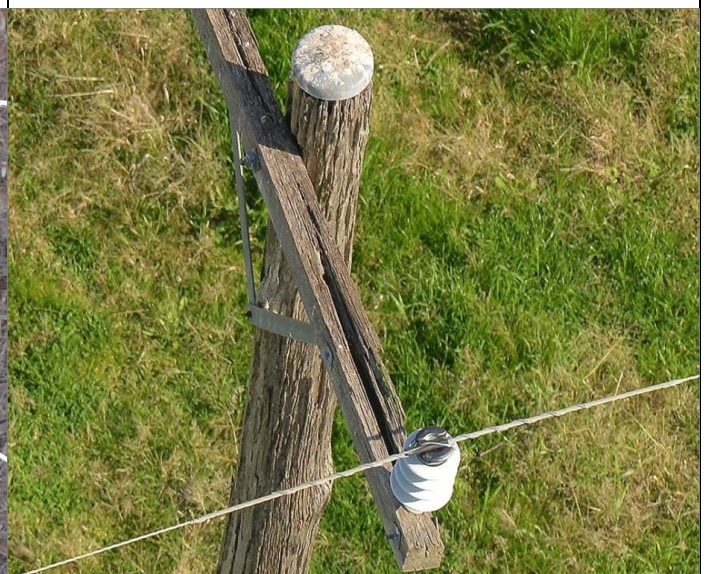
Crossarm deteriorated, deep crack, weathered– A3 task
