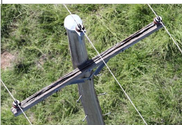
Crossarm deteriorated, severe weathered cracks – A3 Task
