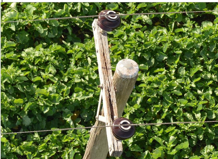
Crossarm deteriorated – A3 task
