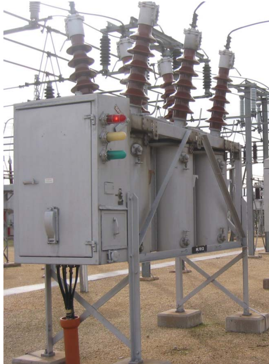
Figure 2 - GEC type LG4C 66kV circuit breaker
