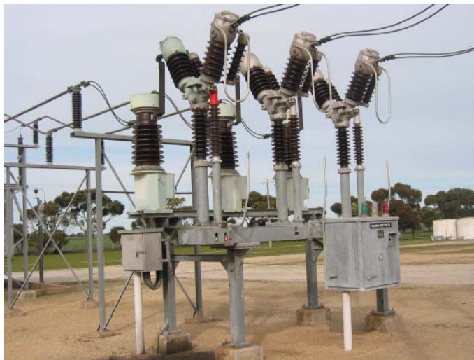
Figure 3 – S&S Type 509 circuit breaker
