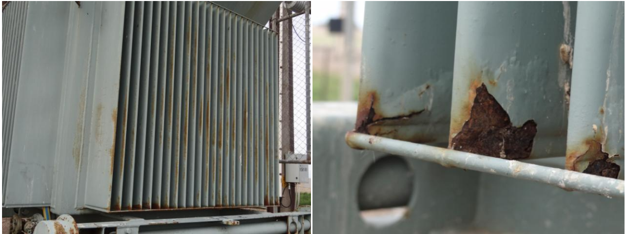
Narrung Substation 2013 33/11kV 1500kVA ST24017 YOM 1999 Installed 1999 ABB QT299
