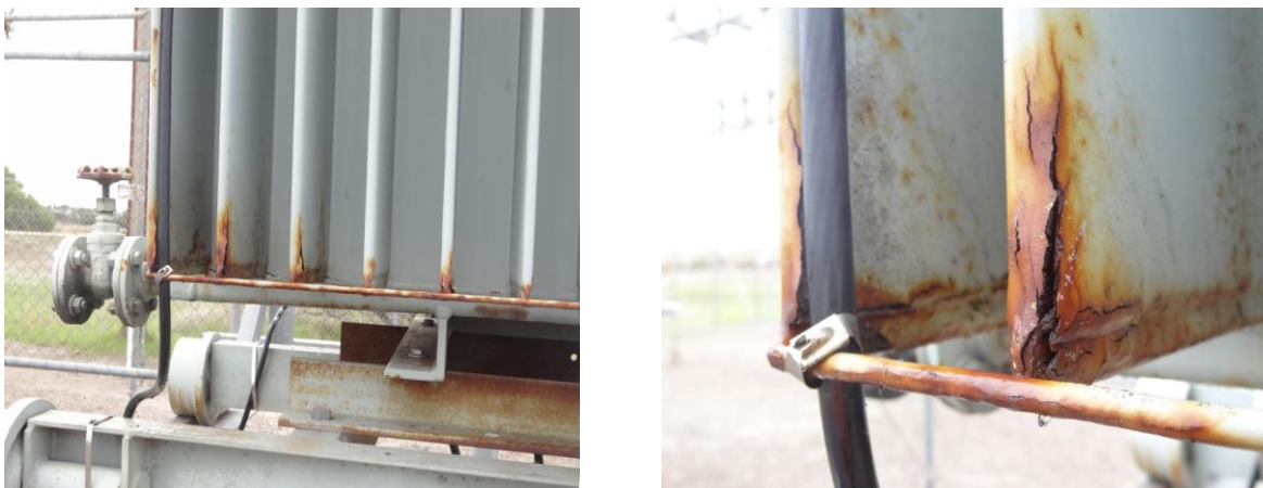
Campbell Park Substation 2013
