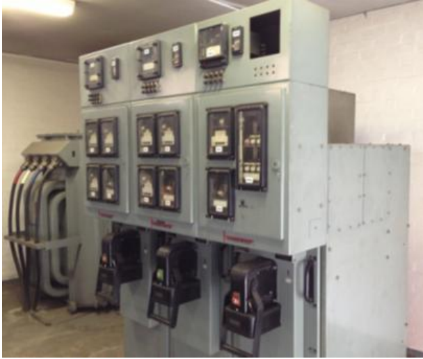
Figure 1 – English Electric oil filled switchgear.
